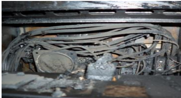
An old electric Frymaster control panel. The fire started below the control area. Note: the supply power connection in the control bay. Typically the high power lines are limited to the outside of control area - this area usually has low power circuits. A loose lug can arc and could have been the source of ignition.
