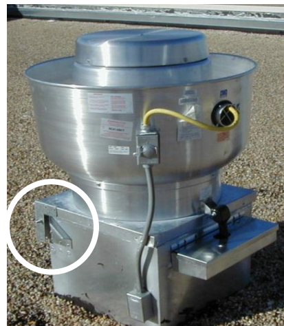
Photo of properly installed, hinged aluminum upblast fan
