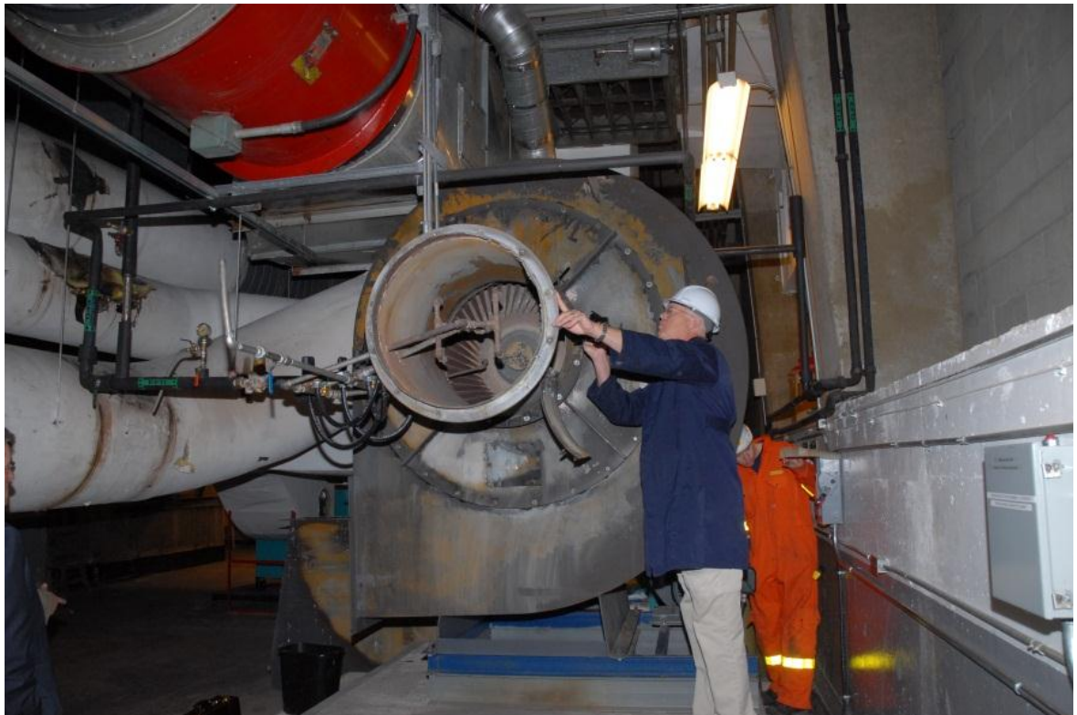
Author examining a large utility fan after a fire
